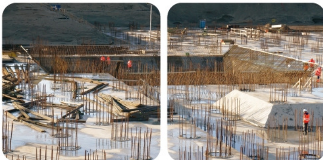
Foundation offsets under boiler plant's piles
